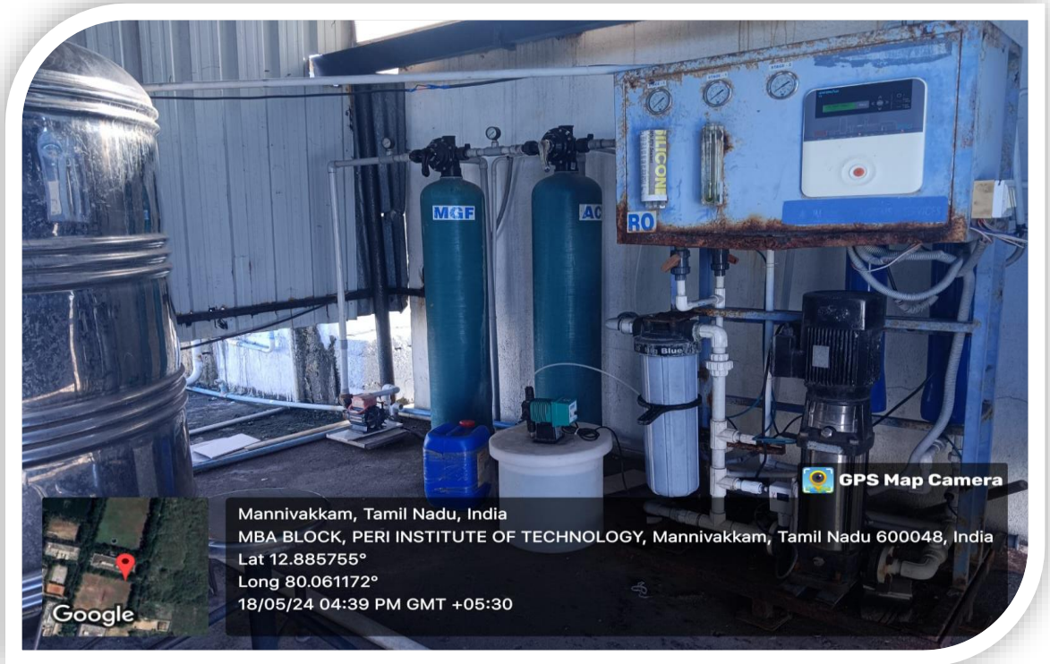
Sewage Treatment Plant
